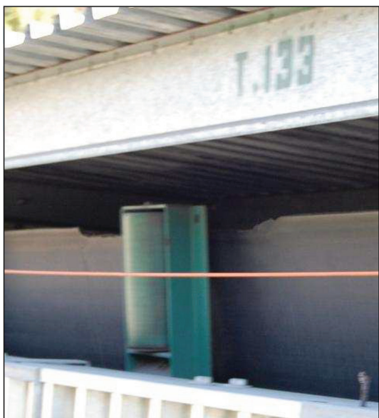
Figure 5 — Edge damage caused by excessive side travel in horizontal curves.
