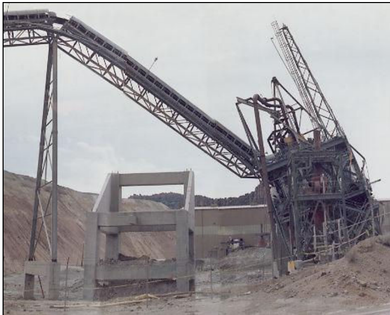
Figure 14 – Structural Failure resulting from dynamic shock waves
