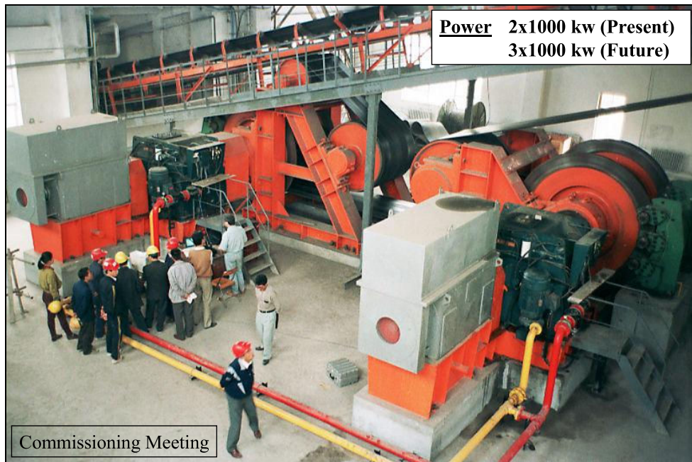
Figure 19 – CST Controller installed in China
