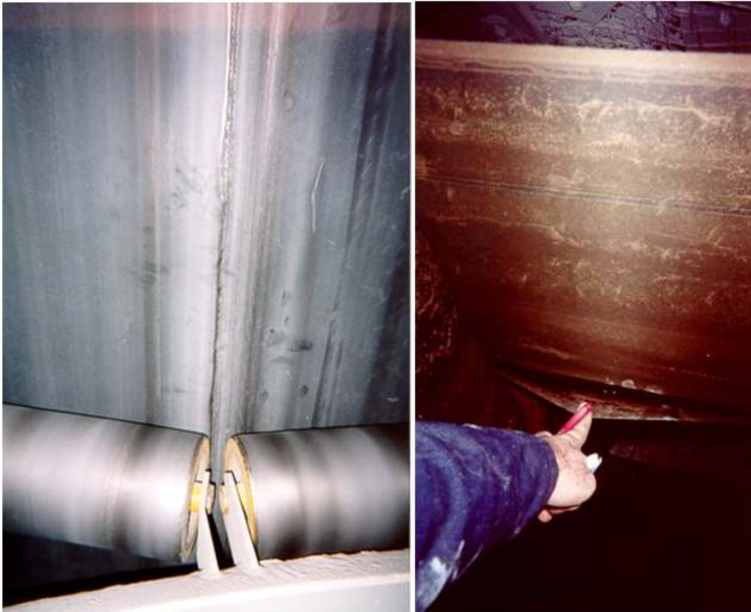
Figure 2. Idler Junction Cover Failure
