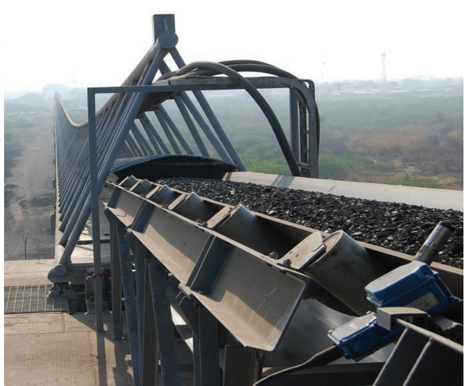
Dust capturing hood designed to shield the coal from wind.
