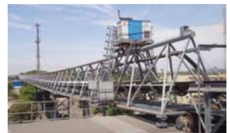
Fig. 6: The maintenance trolley allows personnel access to the conveyor.
