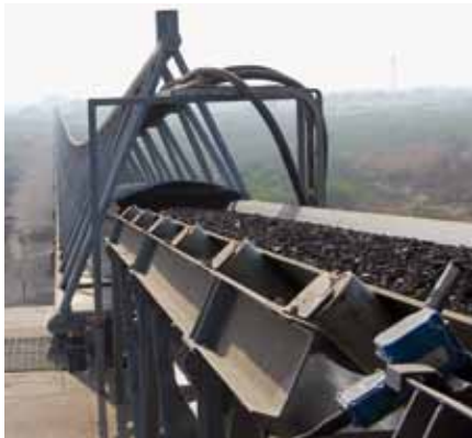
Fig. 7: The belt trough-stringer-hoodcover shields the coal from wind.
