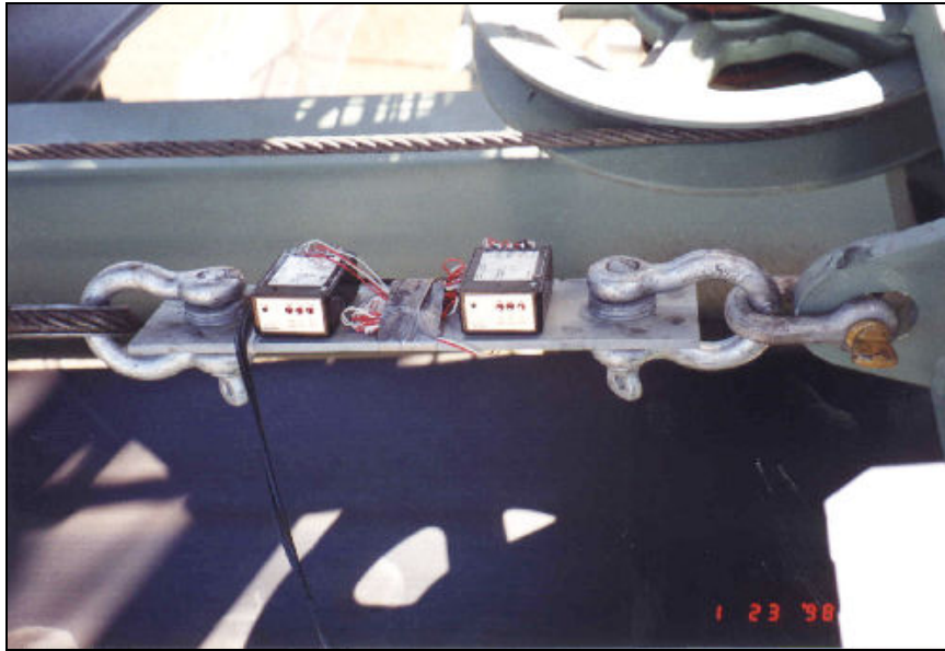
Figure 9: Load cell installed on gravity take-up system
